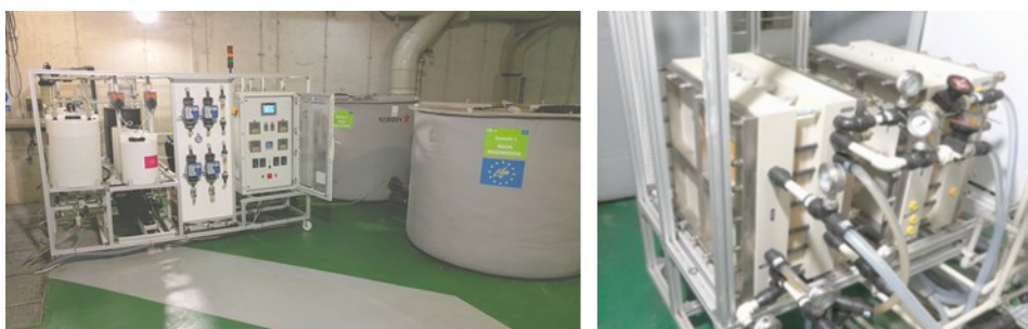
Figure 1. Photograph of the pilot plant (left) and the RED modules (right) used in this study.
